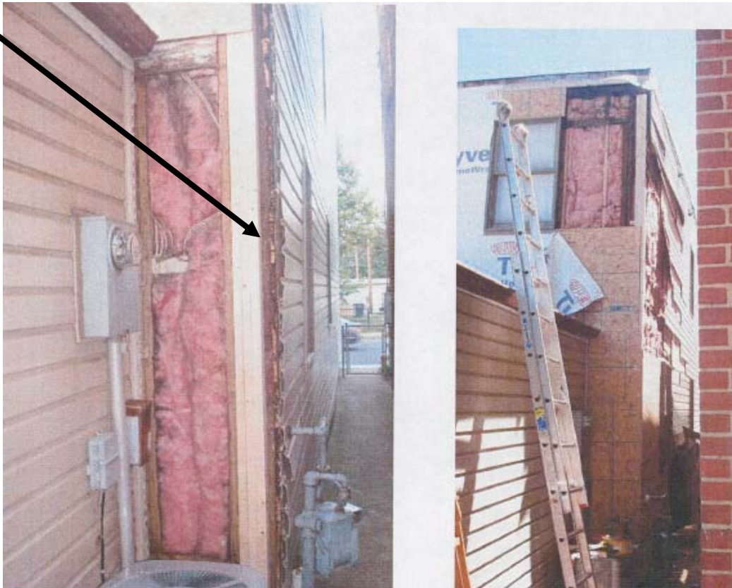
Figure 5: View of Wood and Vinyl Siding Being Removed on the Main Building Mass
