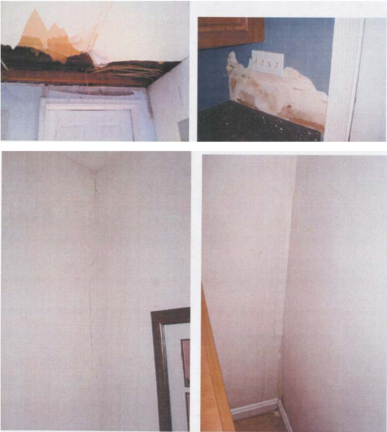
Figure 3: Photos of Interior Water Damage to House after July 2011 Storm
