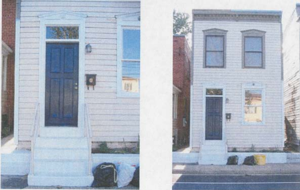
Figure 1: Photo of Front Elevation of the House with German Profile Wood Siding
