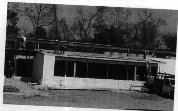
Vola Lawson Animal Shelter - Construction began last spring on the City's new animal shelter on Eisenhower Avenue near Cameron Run Park. The 11,000 square foot shelter will open in early 2002.
