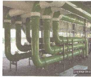
Air Piping for Biological Nutrient Removal Process
