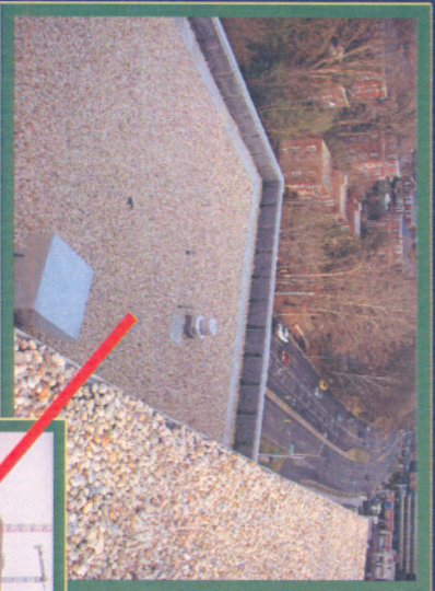
The green roof system was constructed over the existing ballast stone roof.
