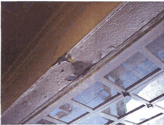
Overhead doors issues
