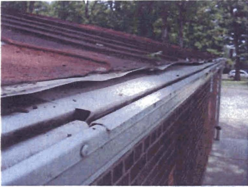
Poor metal roofing conditions
