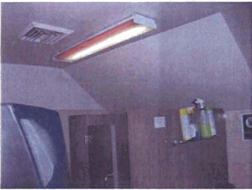
Poor lighting conditions
