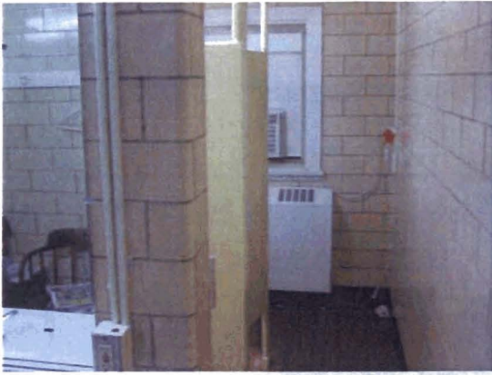
Poor restroom conditions
