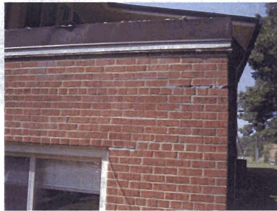
Masonry repair required
