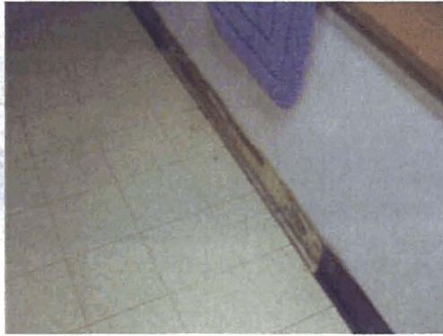
Poor finish conditions
