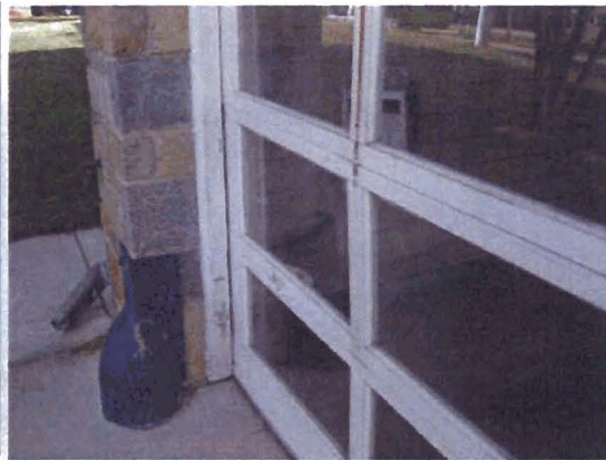
Poor exterior door conditions
