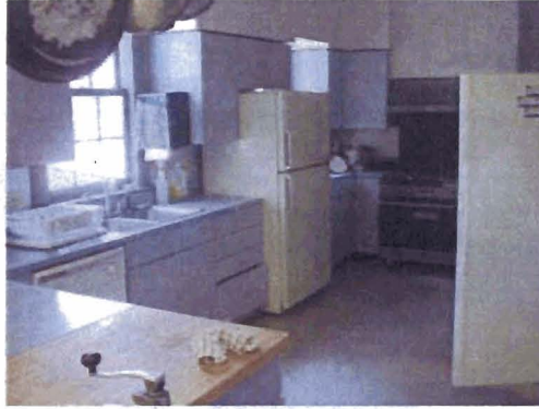
Kitchen renovation required
