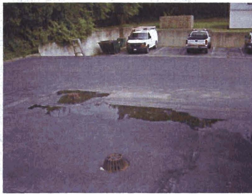
Roof ponding conditions
