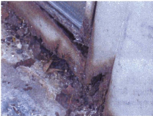
Poor window conditions
