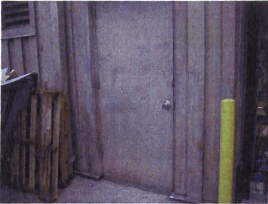
Poor exterior conditions
