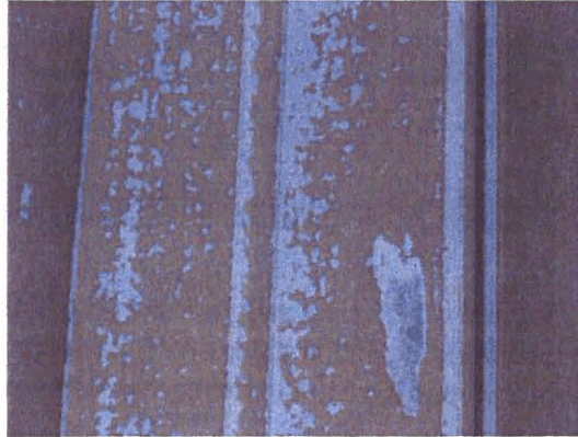
Poor exterior finishes
