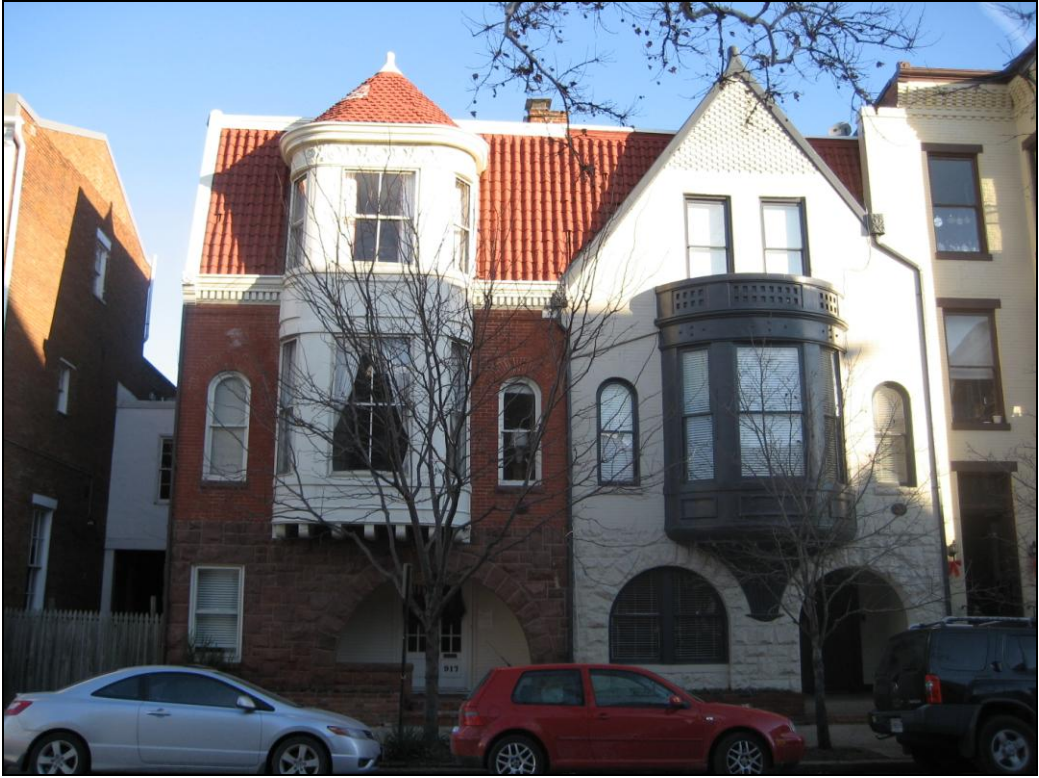
Figure 1. Front elevation of 917 Prince Street (on left) with turret with existing clay tile roof.
