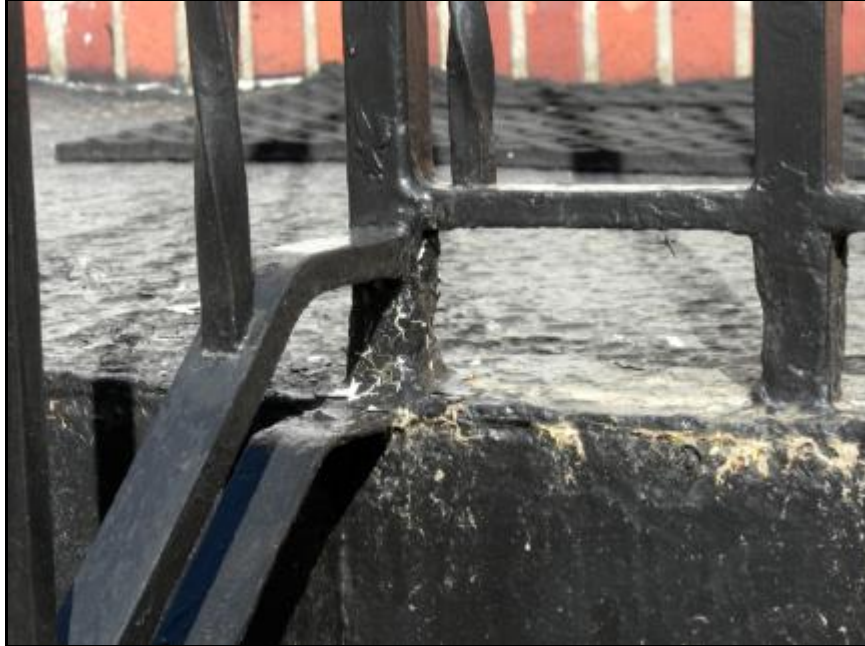
Figure 3. Rust on existing iron deck at 821 S Lee Street.
