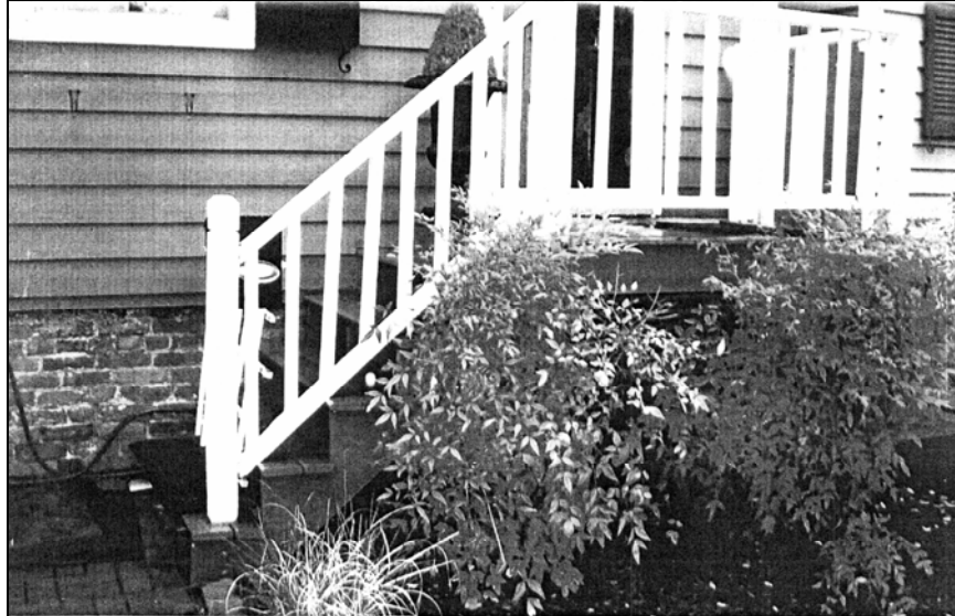
Figure 1. Existing deteriorated wood porch.
