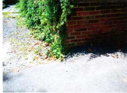
3: VIEW AT REAR OF PROPERTY GRADE CHANGES BEGIN AT CORNER LOT LINE AND GROUND DECLINES TOWARDS PUBLIC UTILITIES.
