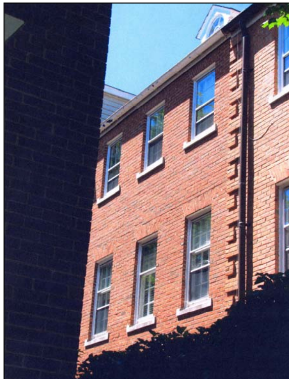
Figure 2. Rear (east) elevation of 602 South Lee Street as seen from Gibbon Street.
