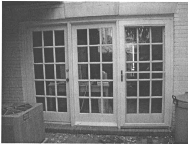
621 Pommander Walk: Rear Window Wall Replacement: same material, same design, same color
