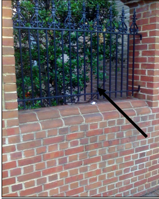
Figure 1. View of south wall of 219 South Royal Street showing approximate location of proposed vent.
