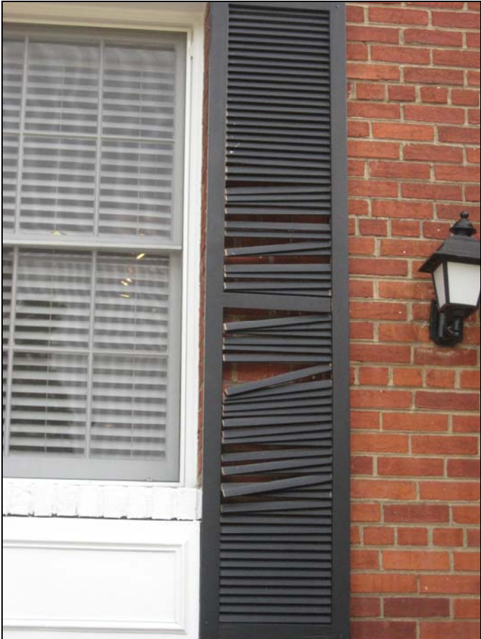
Figure 4. Detail of existing deteriorated wood shutter.
