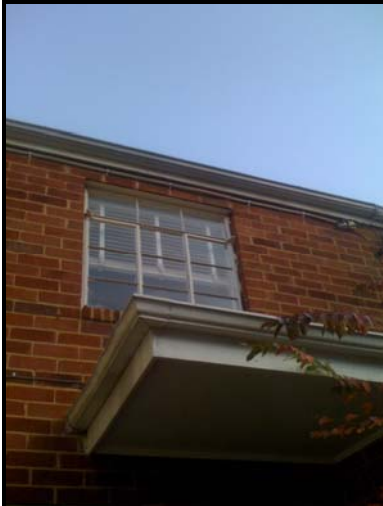
Figure 4: Existing Metal Single Pane Window
