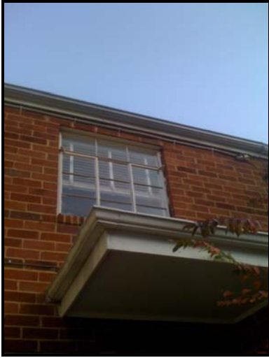
Figure 4: Existing Metal Single Pane Window
