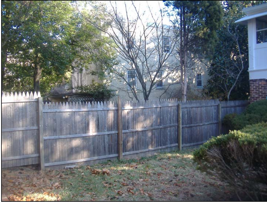
Figure 6. Existing wood fence to be demolished and stepped down in height according to grade.
