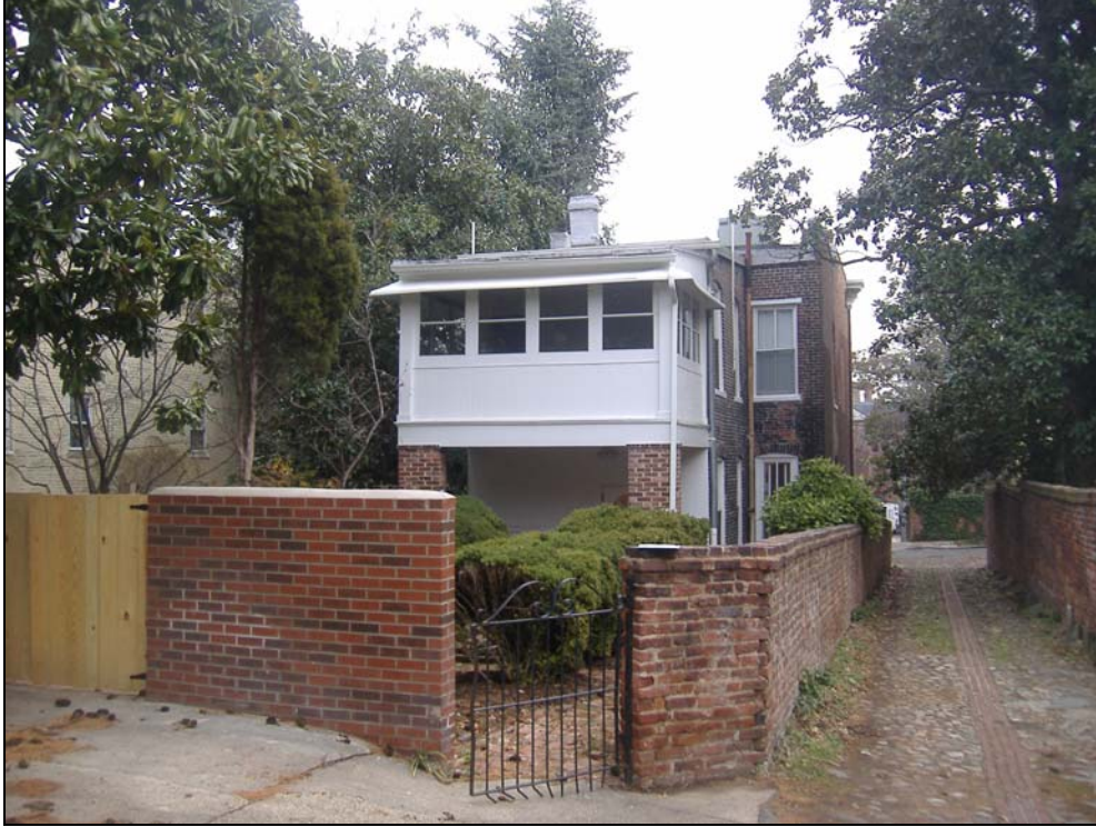
Figure 4. View showing non-historic brick wall adjacent to parking area and historic brick wall on alley.
