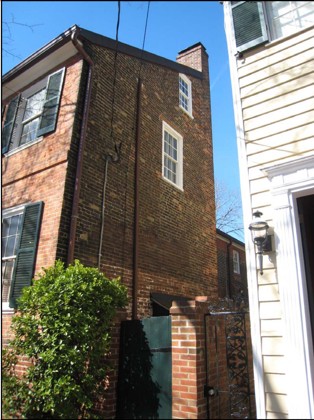
Figure 5: Photo showing flounder side of 210 North Fairfax Steet
