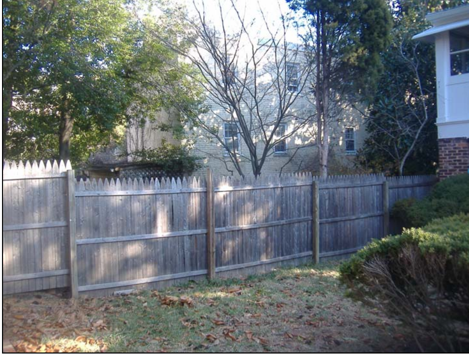
Figure 6. Existing wood fence that steps down in height according to grade and is proposed to be demolished.
