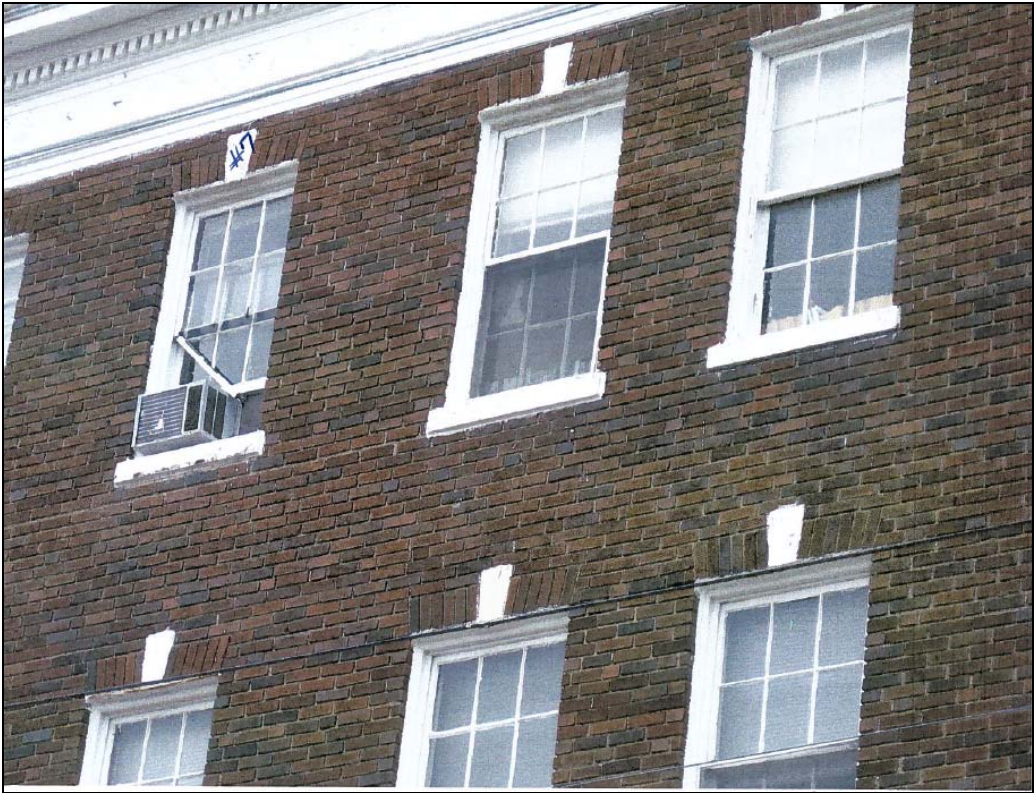
Figure 4. Views of existing windows on north façade showing window labeled #7 that was administratively approved for replacement.
