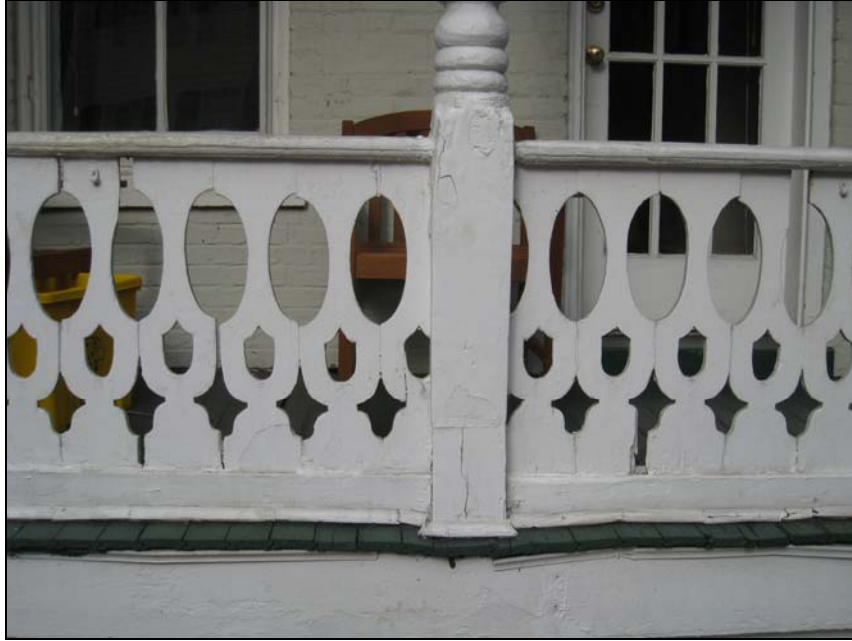
Figure 4. Detail of porch illustrating areas in need of repair.
