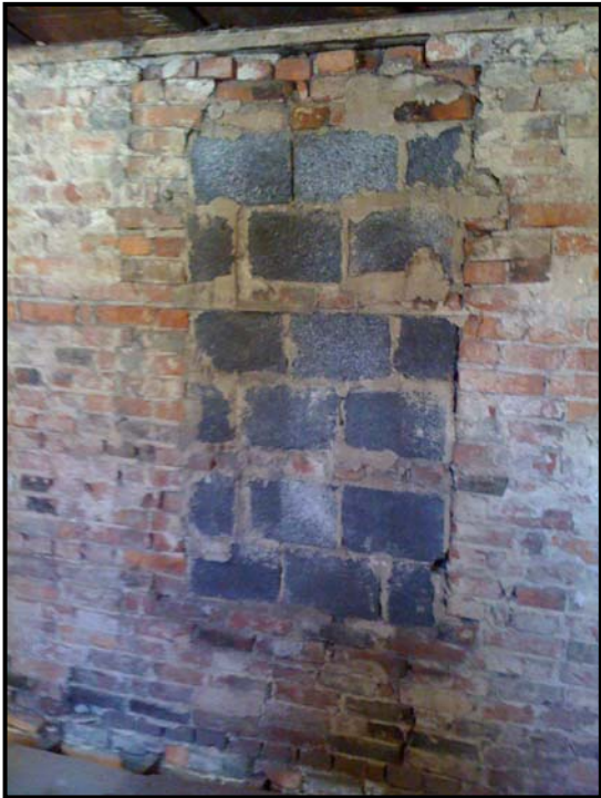
Figure 17: View of original second floor window to be enclosed with brick and shutters
