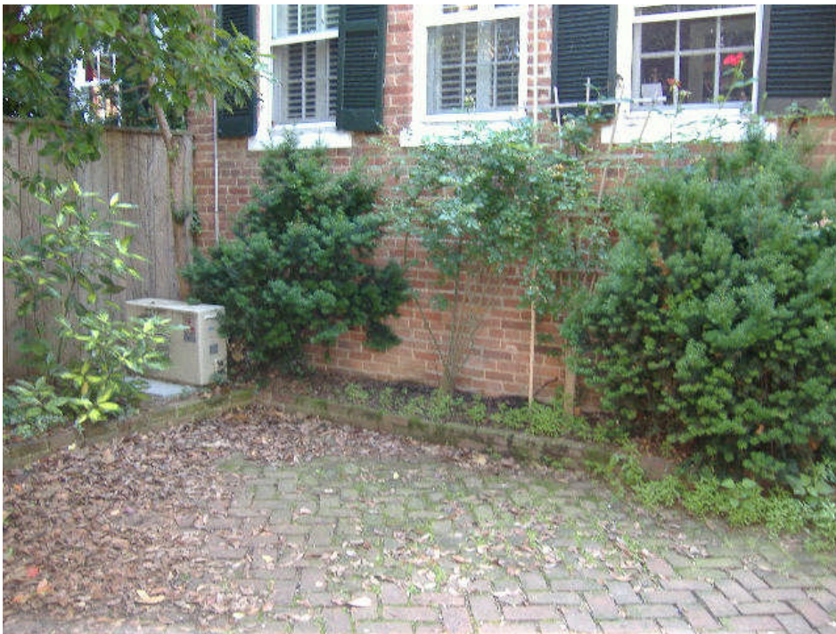
Figure 4: Detail View of Location of Generator
