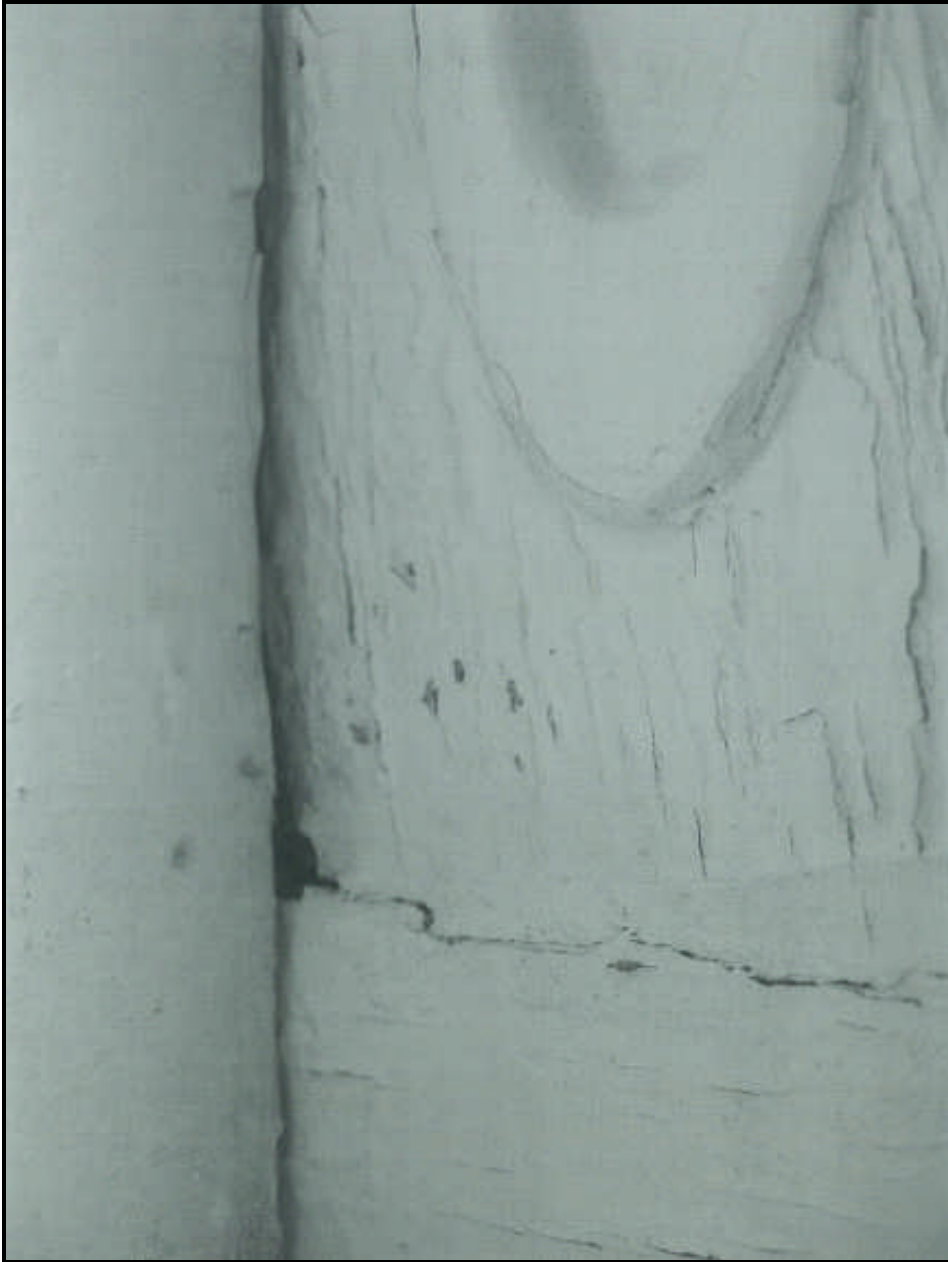
Figure 9. Window Survey: Existing Conditions-Exterior Paint Conditions: Typical
