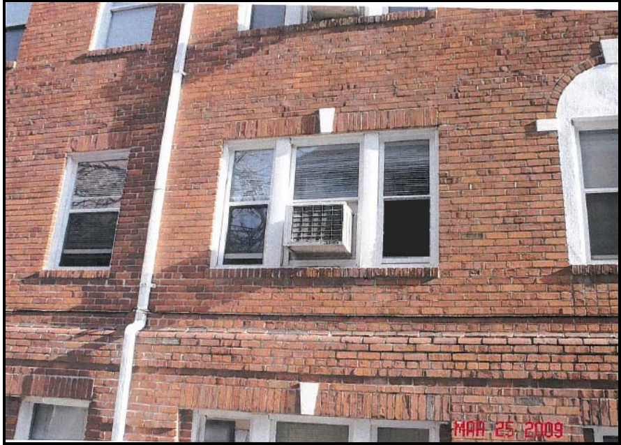
Figure 2. Photograph of building with existing HVAC units.
