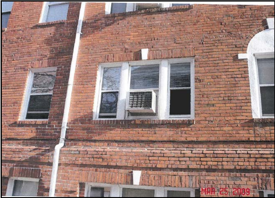
Figure 2. Photograph of building with existing HVAC units.
