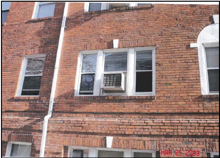
Figure 2. Photograph of building with existing HVAC units.
