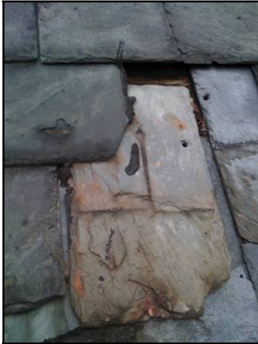
Figure 11: Photo of damaged slate.
