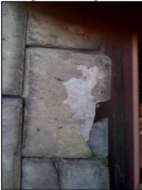
Figure 12: Photo of damaged slate.
