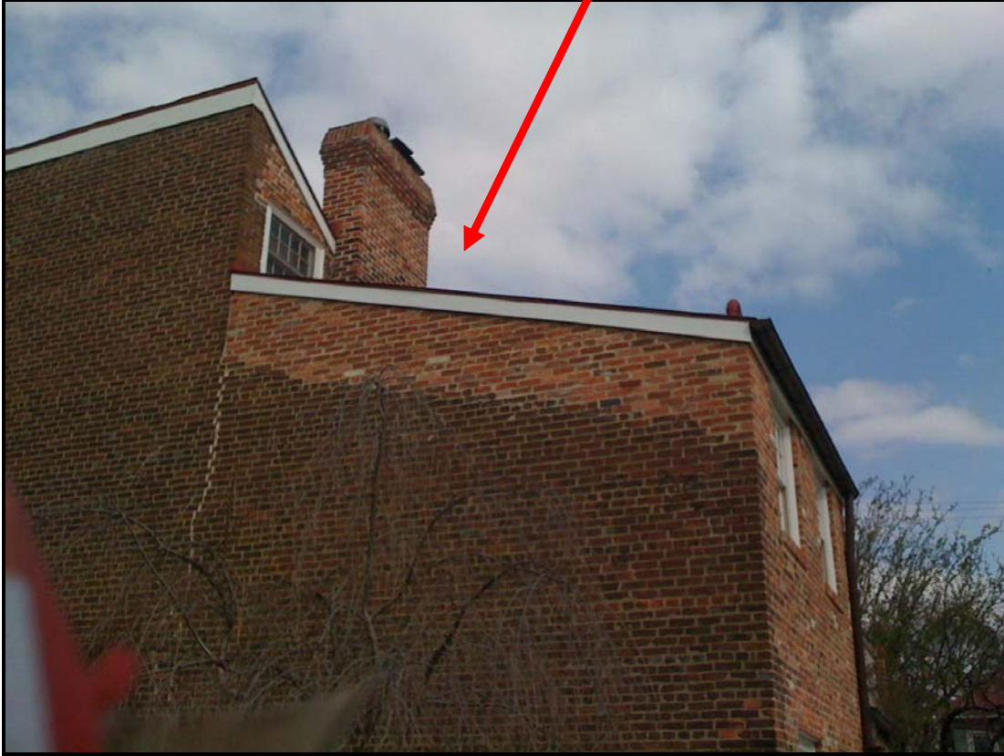
Figure 3: View of rear addition showing new brick from previous alteration
