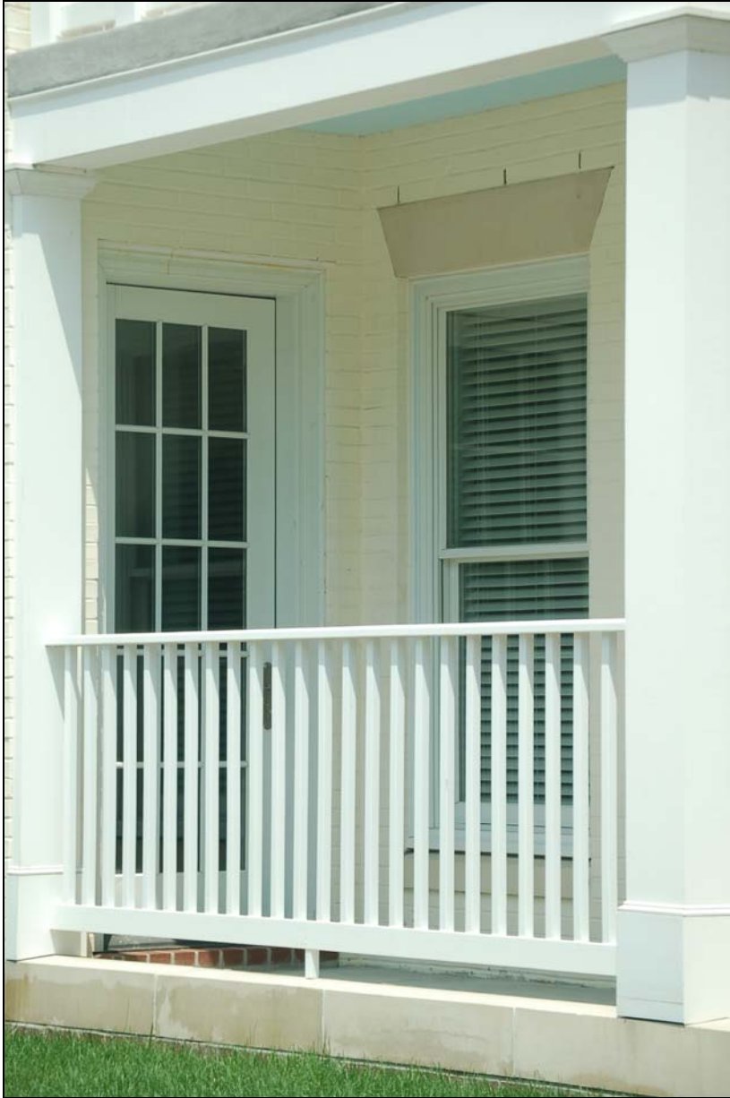
Figure 3. Railing on North Columbus Street.
