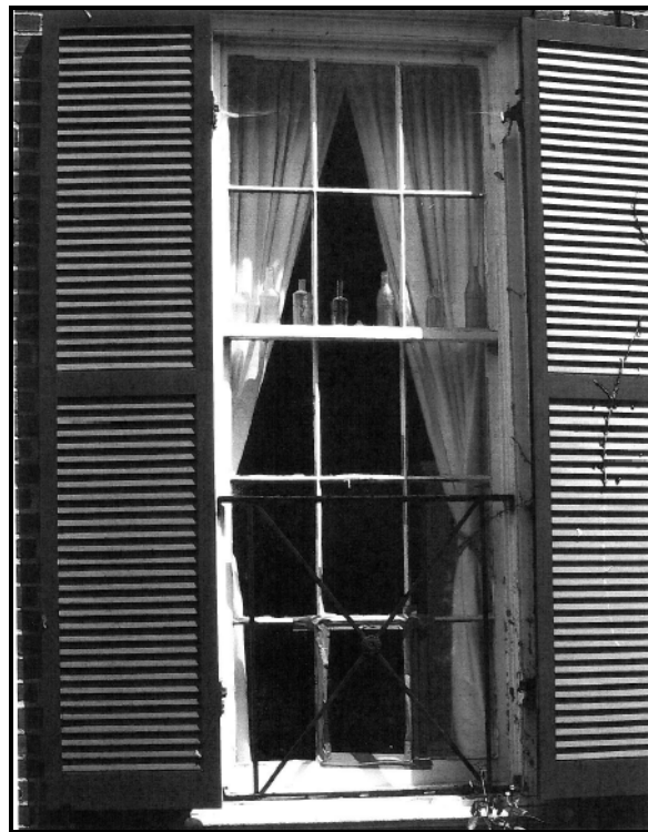
Figure 2. Photo of damaged window.
