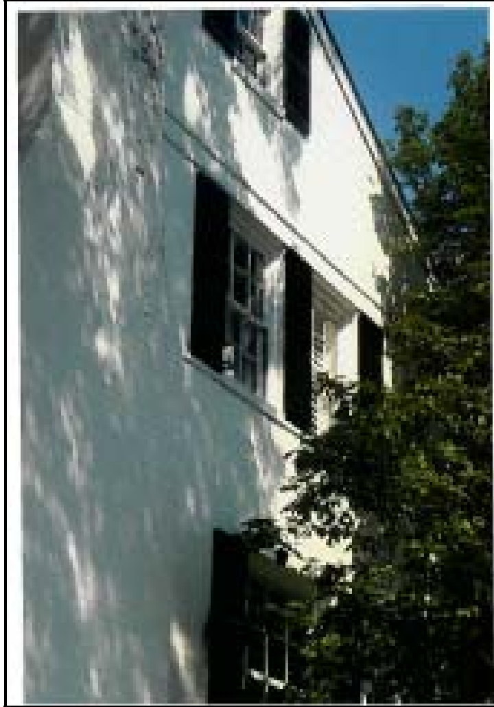
Figure 3: Second floor windows to be replaced
