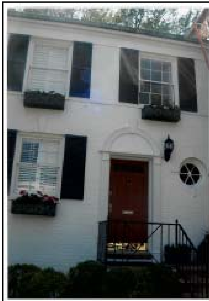
Figure 2. Second floor windows to be replaced
