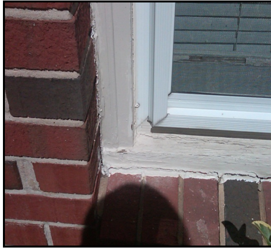
Figure 5. Existing Windows Condition
