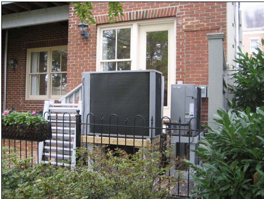
Figure 2. 17 Keith's Lane showing replacement HVAC units on platforms without screening.
