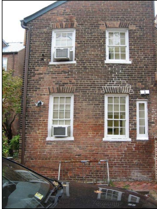
Figure 3. Rear (east) elevation.
