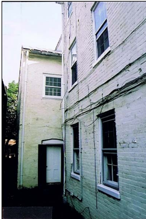
Figure 2. Rear (west) elevation of main block and side (north) elevation of rear block.
