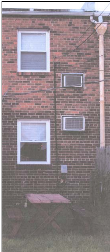
Figure 2: Example of through-the-wall AC units
