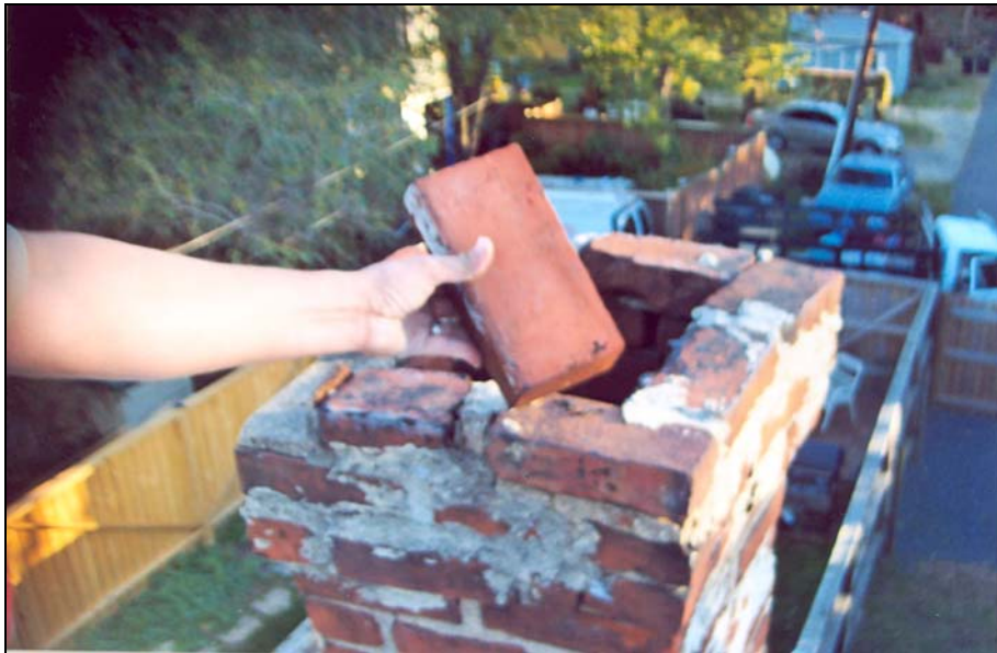
Figure 4. Detail of damaged chimney.
