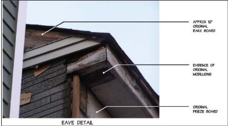
Figure 15. Evidence of original modillions for replacement.
