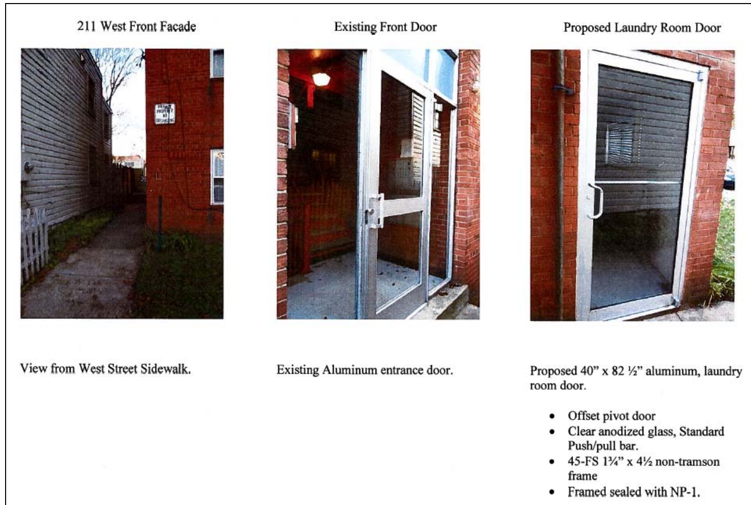
Figure 1. Photographs of portion of front elevation as viewed from North West Street, existing aluminum and glass entrance door, and newly-installed aluminum door in new opening.
