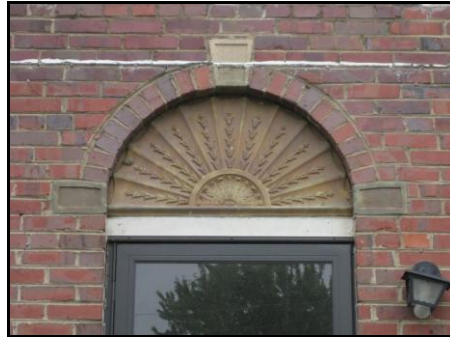
Figure 1: Cast concrete door architrave and the ghost marks from the metal awnings at 1603 Princess Street.
