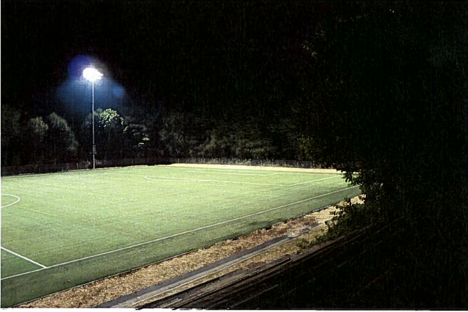
Sample Field Lighting with Low-Spill Technology at Fort Ward Field
