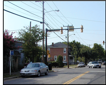
Overhead Utilities on Columbus Street
