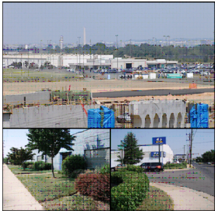
Figure 13. Existing Site Conditions (Top: View south with new Route 1 Bridge in the foreground; Bottom: Views west of Route 1)
